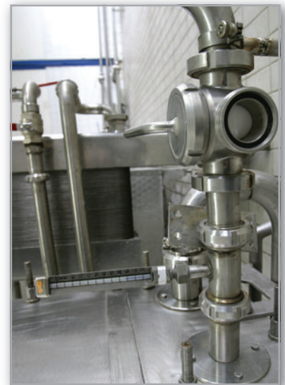
Control Systems (p. 308)
